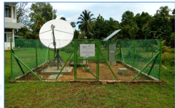
Stesen AWS Betong, Sarawak AWS Station Betong, Sarawak
